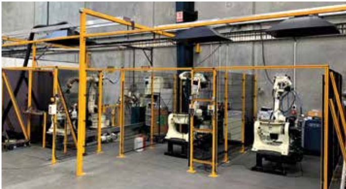
Line-Up of Turn-Tilt Robotic Welding Cells
